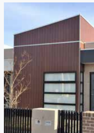
COMPLETE: After 3 coats the timber is restored and is now UV protected.
