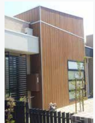
4 MONTHS: The board shows signs of lightening.
