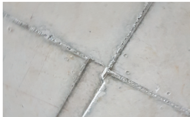
Misaligned formwork was identified as a contributing factor to tension in internal framing.
