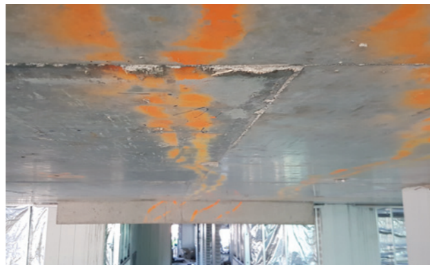
Formwork residue and concrete debris often present uneven fixing surfaces which are not made good prior to wall installation.
