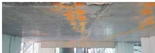
Formwork residue and concrete debris often present uneven fixing surfaces which are not made good prior to wall installation.
