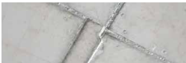
Misaligned formwork was identified as a contributing factor to tension in internal framing.
