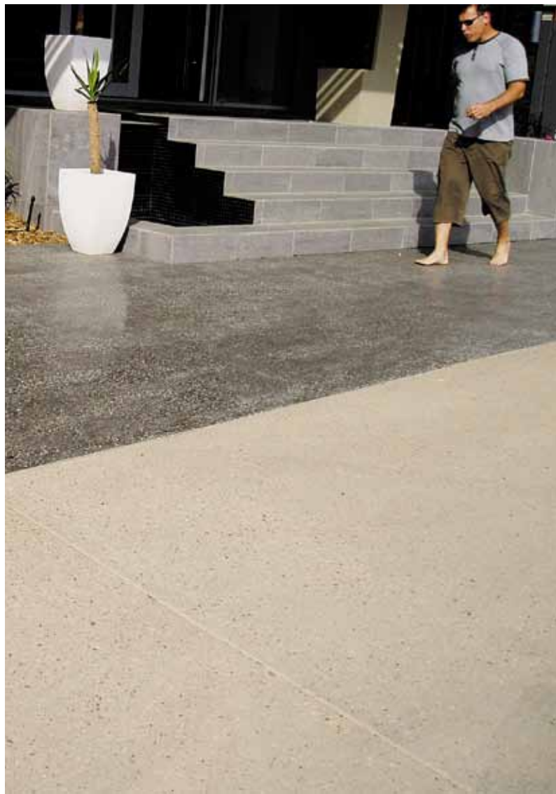
Above: A stunning contrast with honed and polished concrete. Colours: CCS Black 21 and CCS Driftwood.
