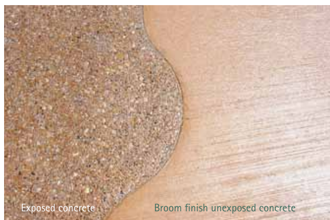
The same colour was used on both sections of this concrete. Note how 'exposing the concrete' gives a completely different colour appearance.
