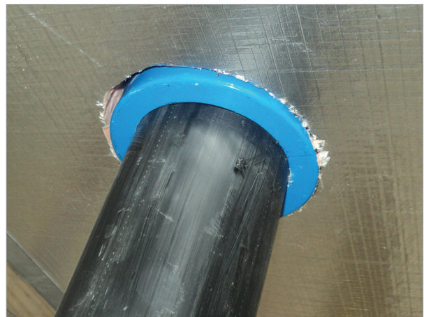
Figure 7. Penetration example - Kingspan Kooltherm® K10 G2 Soffit Board installed tight around the fire collar and HDPE service pipe.
